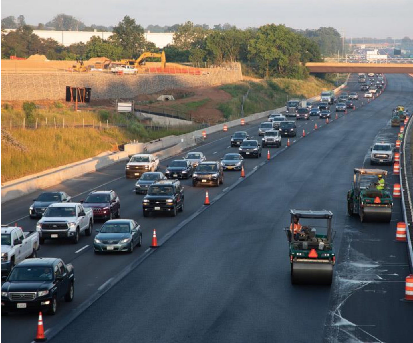
The alignment includes new asphalt pavement and recycling of rubblized concrete. Photo courtesy of EMP
