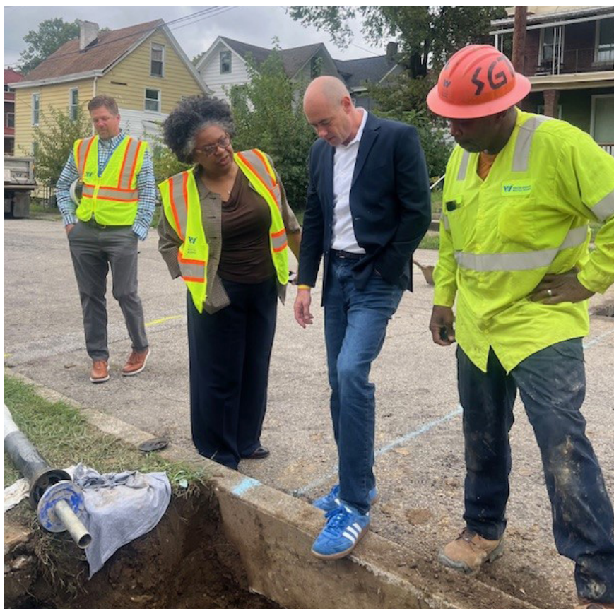
Cathy Bailey shares and explains the lead line replacement process to Ohio Congressman Greg Landsman during a site visit in Cincinnati. Photo credit: Greater Cincinnati Water Works
